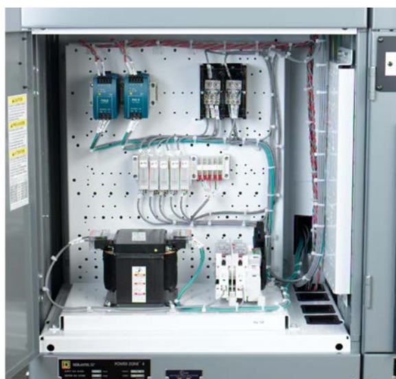
Figure 14 - Typical Auxiliary Instrument Compartment
