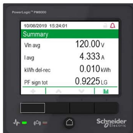
Figure 63 - 3.5" Color Graphic Display (mounted on Main Breaker door n PZ4)
