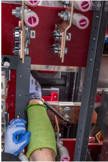
Figure 43 - Rotating Splice Bus
