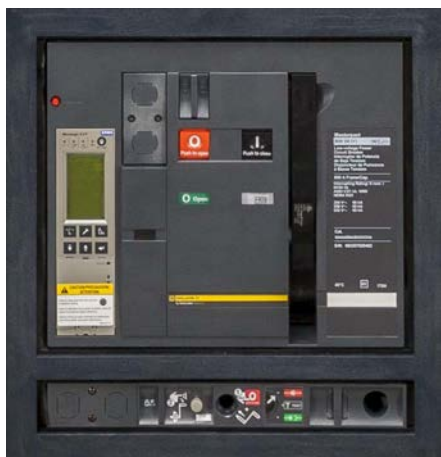
Figure 40 - Breaker Compartment, Door Closed
