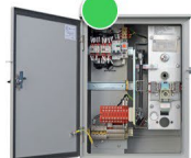
Motor drive Disconnecter drive cabinet
